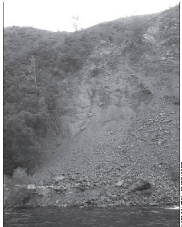
The massive rockfall spills into the Merced River and covers Highway 140.
